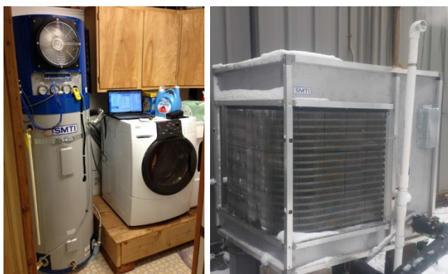
Figure 1. GHP as Water Heater (Left) and Space Heater (Right) Units in Field, in WA and TN
