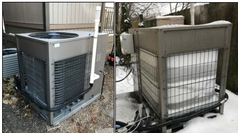
Figure 2: Pilot installations of the Next Gen GHP
